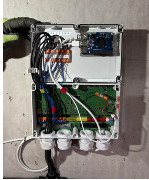
Monitoring data acquisition unit
